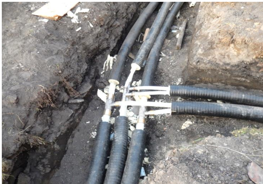
Fig. 3. Laying of the pre-insulated polymer pipes for heat supply networks in the village Namtsy (Namsky district)
